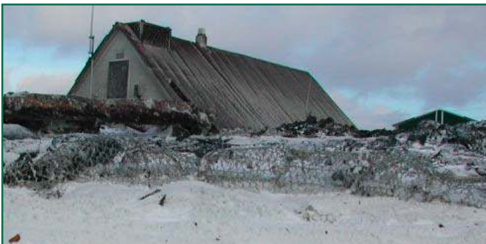
The storm water emptied the gabions in front of the 108 year old church. The gabions are wired mesh that are filled with rock to help protect the land from water damage.
