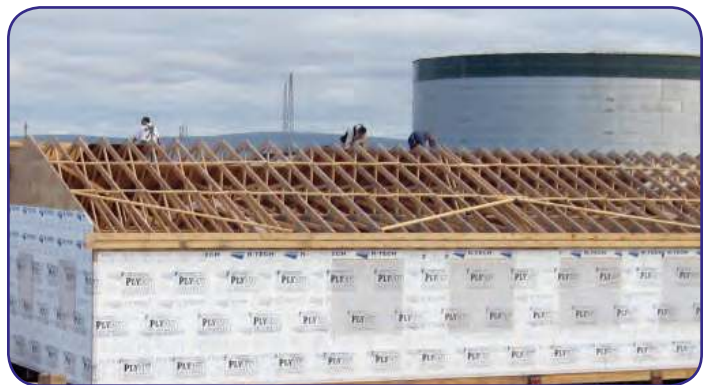
The Teller project of building two duplexes for the Bering Strait School District provided an opportunity for BSDC to employ five local shareholders in Teller, so far.
